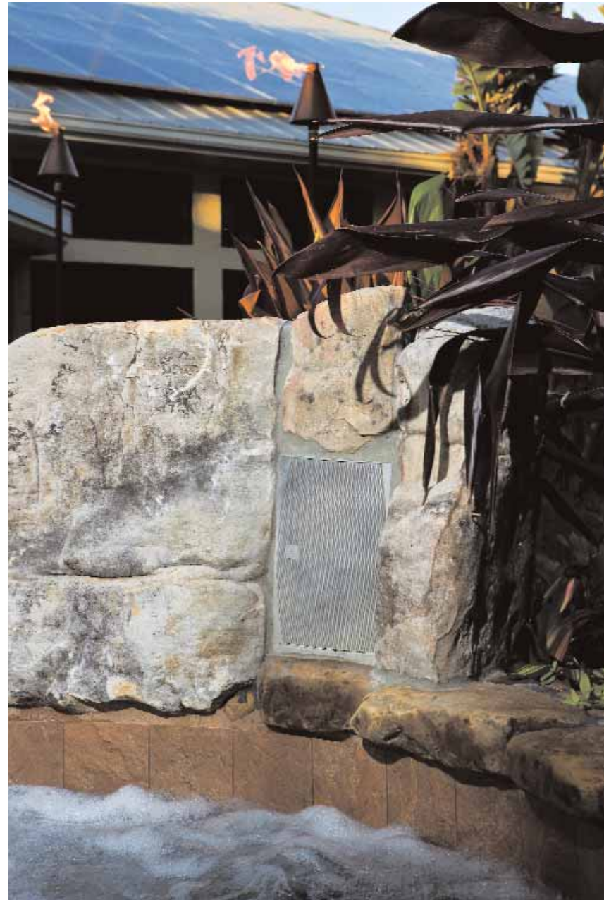
Music to the Jacuzzi in this Florida home flows out of Sonance Mariner 61 speakers that were grouted at the time the stonework was constructed, so the weather-hardy speakers appear to be part of the wall. System design and installation by Advanced Electrical Installations, Punta Gorda, FL.
